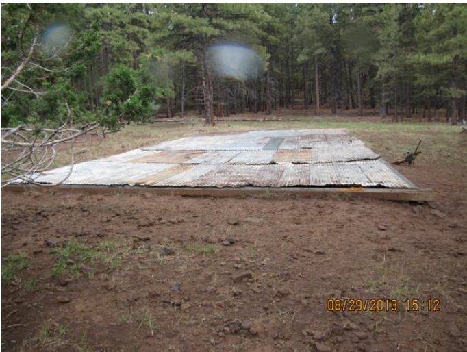
Deteriorated frame and broken apron
