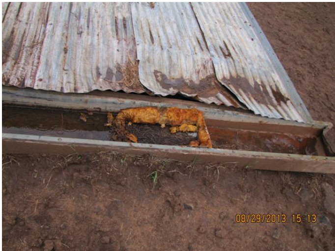
Close up of repairs that have failed
